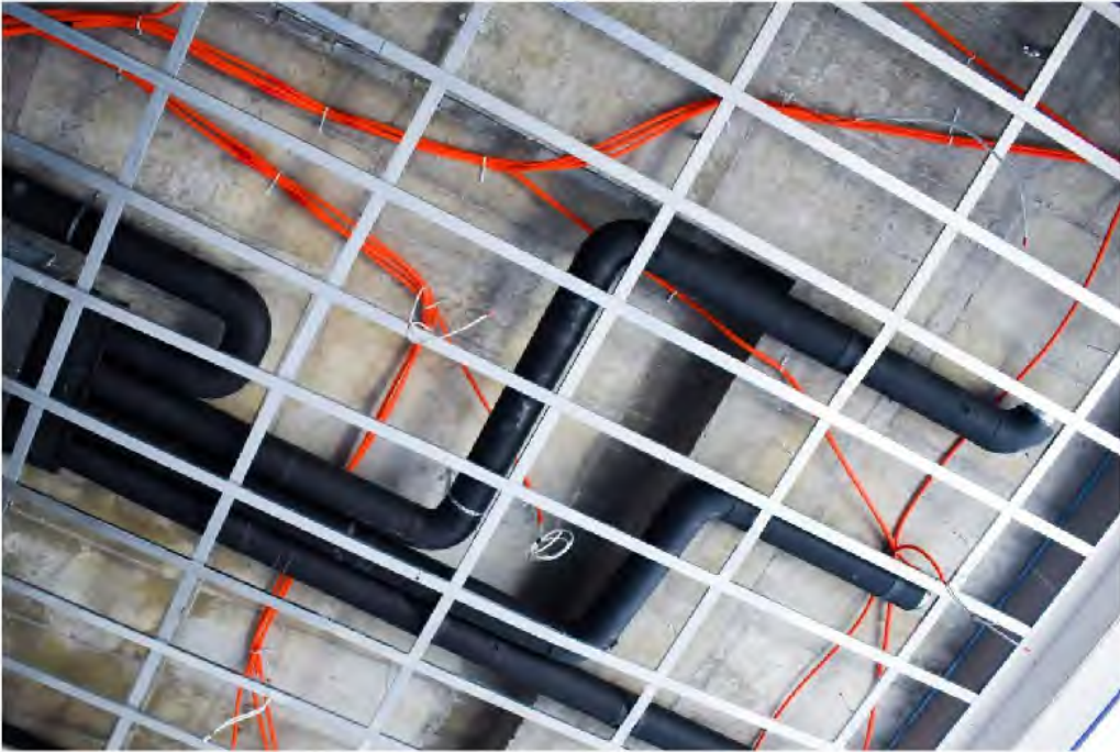
Ducts, Plenums, and Other Air-Handling Spaces
