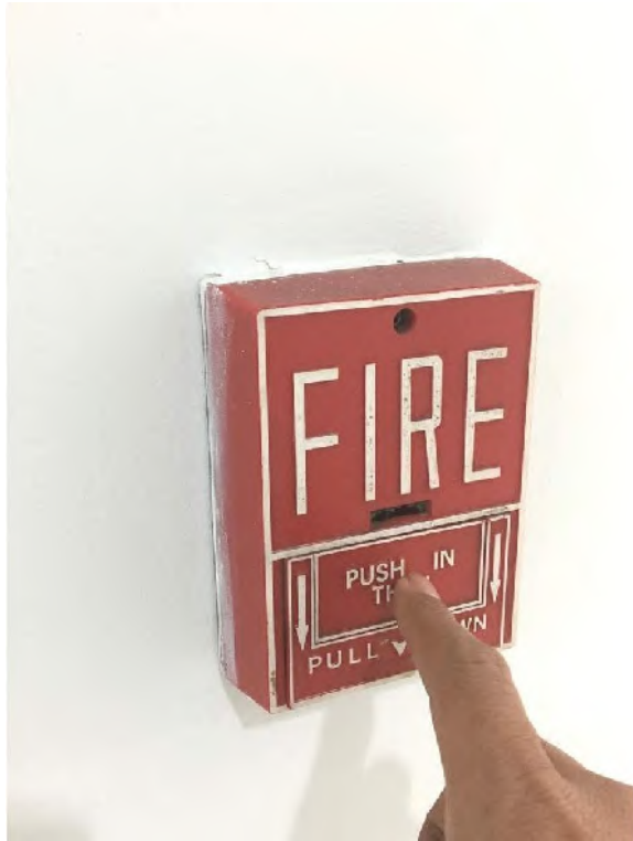
Manual Fire Alarm Boxes
